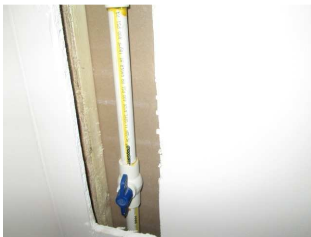
Water main shut off
