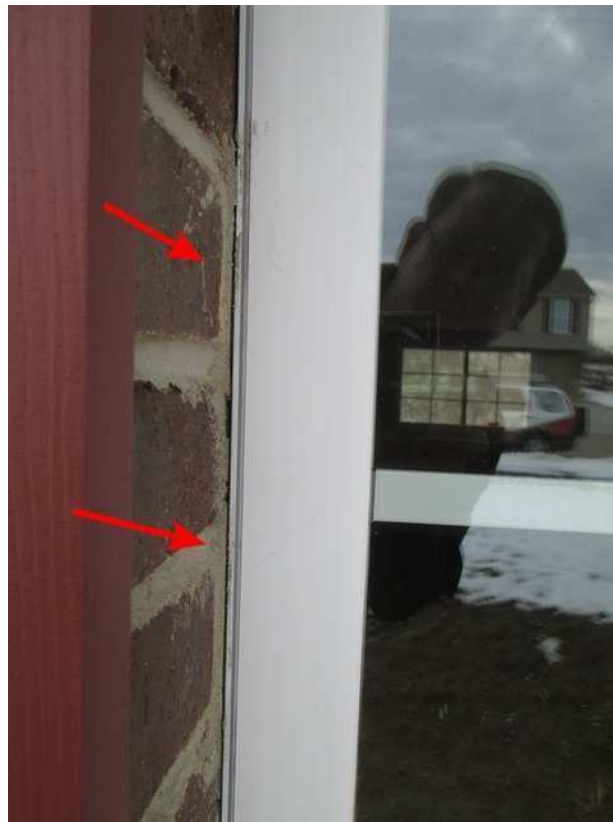
Missing caulk on front lower window
