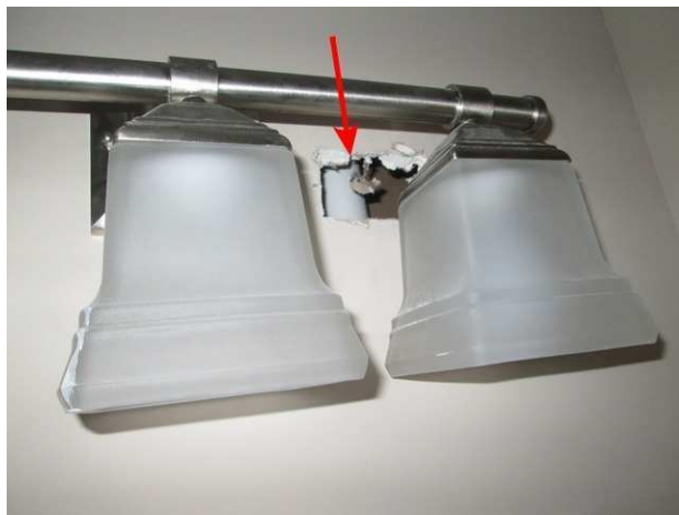
Drywall damage in half bath above sink
